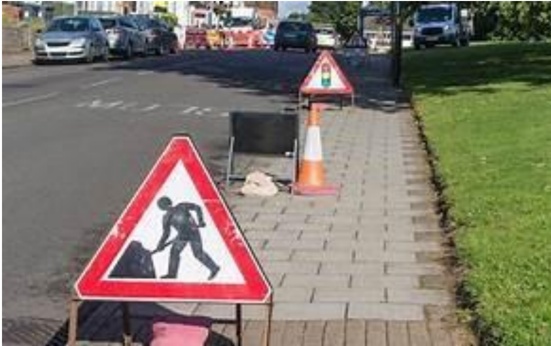
Minor anomalies on signage.
