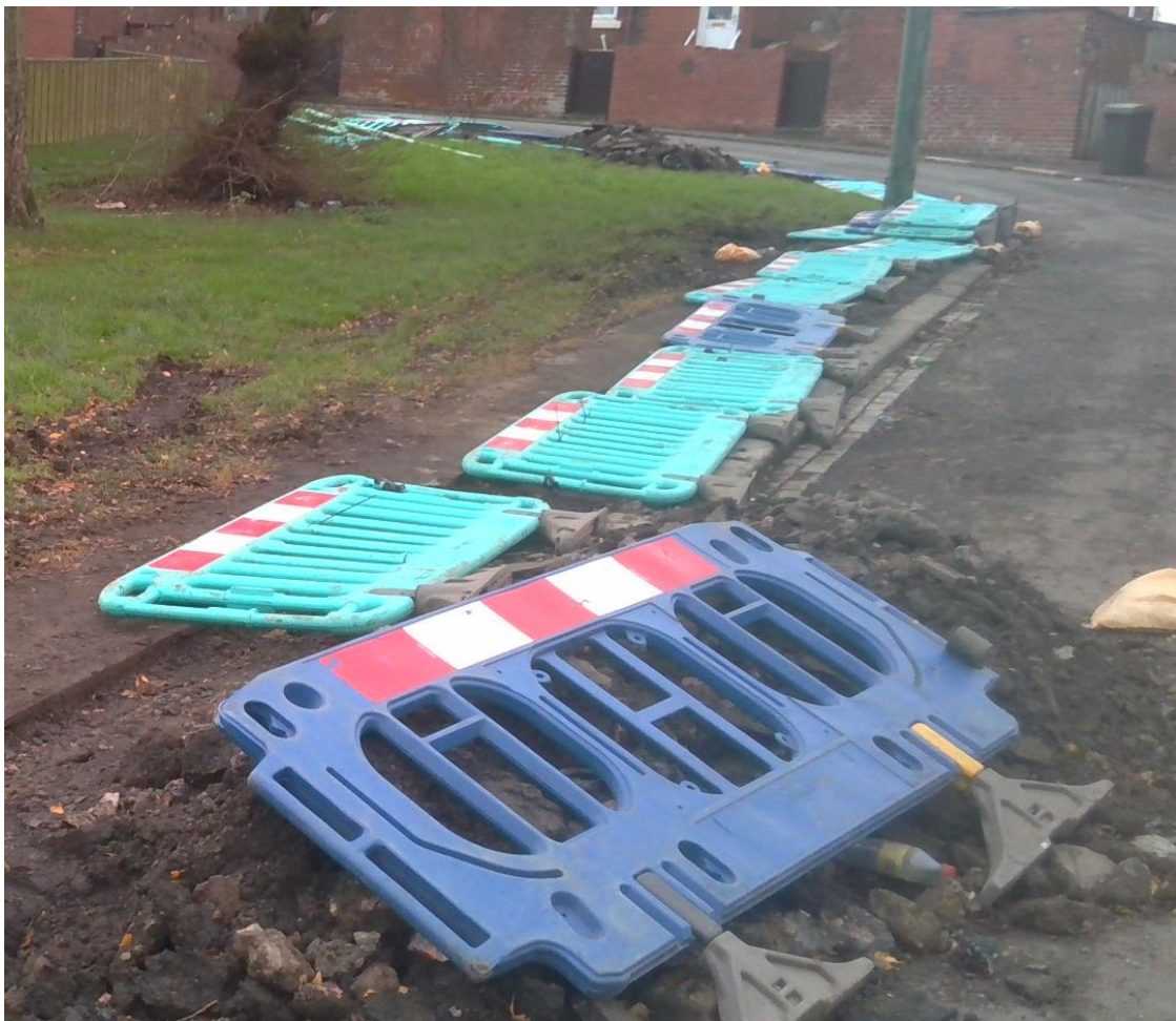
Vandalised unmanned site
